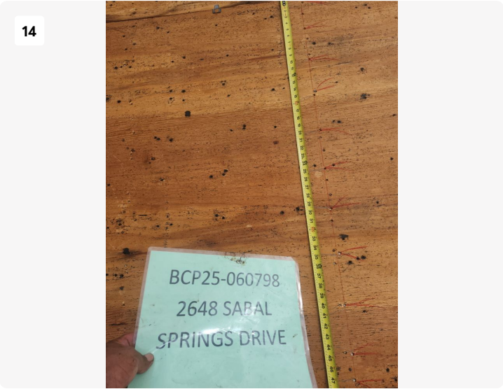
Project: 2648 Sabal Springs Dr unit 6 Date: Jul 2, 2025, 12:50 PM Creator: Lucio Roofer
